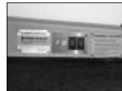
Photo #2 Control Panel
